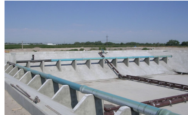
Waste Water Treatment Plant Aeration Basin
