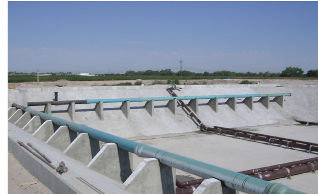
Waste Water Treatment Plant Aeration Basin
